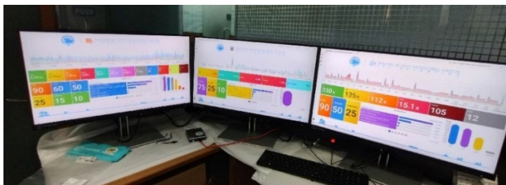
C3iHub SoC Installed at IPA (2022)
